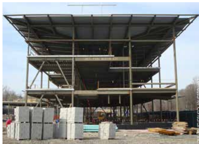
▲ The 8-in.-square HSS columns provided adequate capacity in most cases under load combinations.
